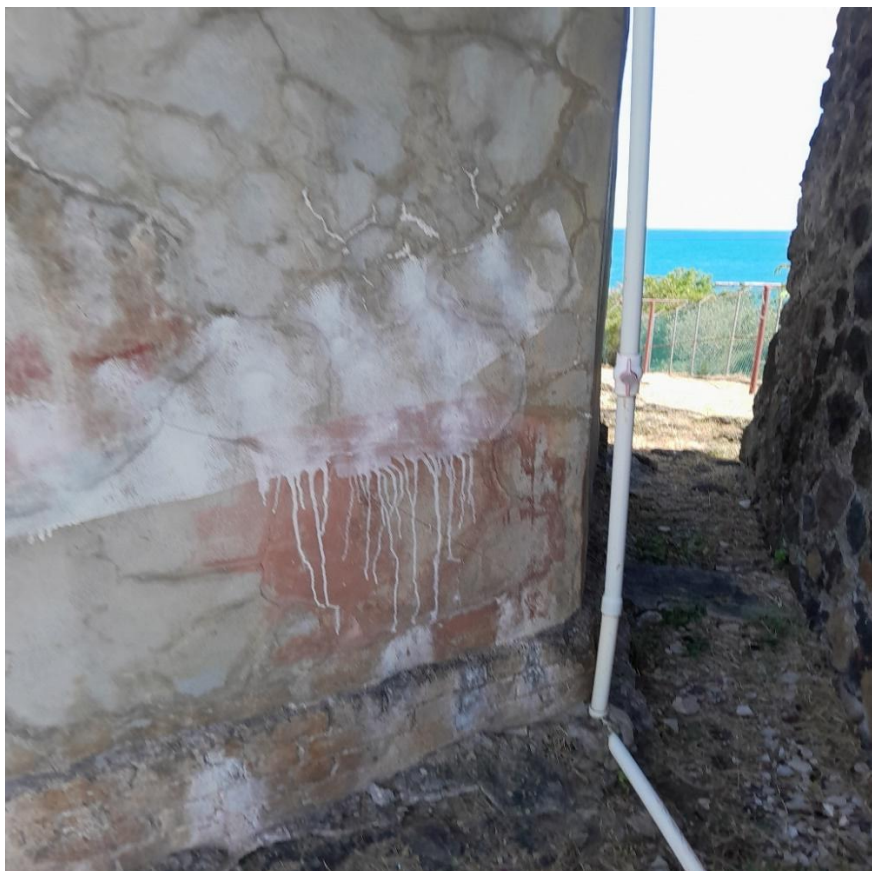
Drain from existing water tank
